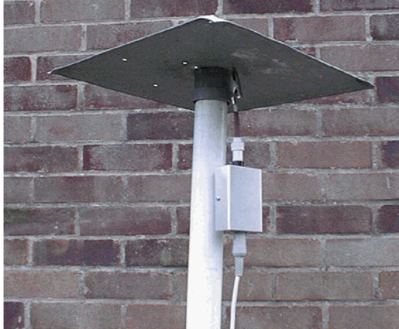
Meter interface unit connected to the sensor probe plate.
